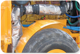
Mining Vehicle, Exhaust & Catalyst Insulated
