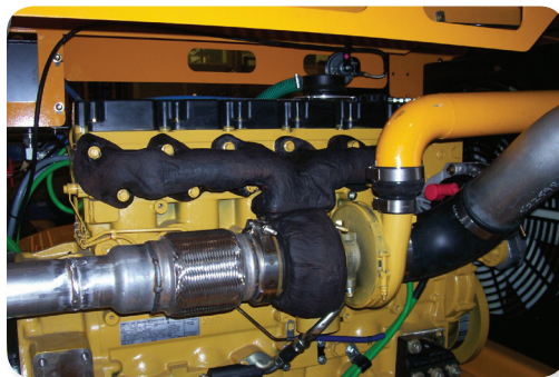
Turbo and Manifold with Firwin Hard Coat insulation
