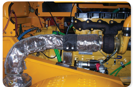
Mining exhaust with both MineWrap™ and Hard Coat
