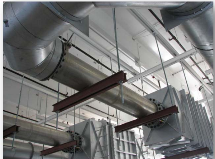
SCR System, without Insulation Blankets
