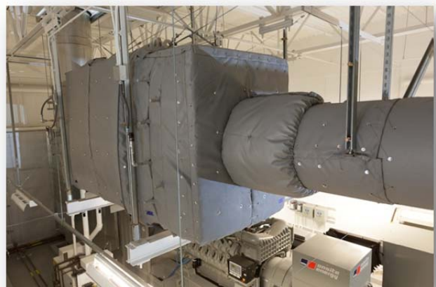
SCR System, Removable Insulation Blankets Installed
