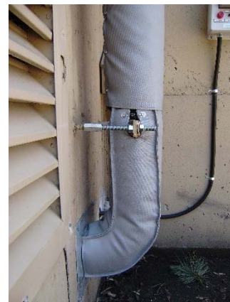
Pipe Bracket / Protrusion
