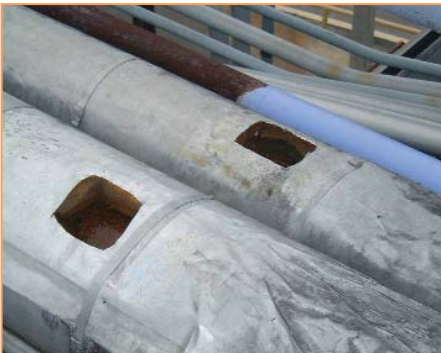
Figure 3: These rooftop lines have unrepaired access in a "catch rain" position.
