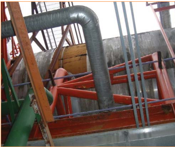
Figure 5: This jacket and vapor retarder were damaged by weather.
