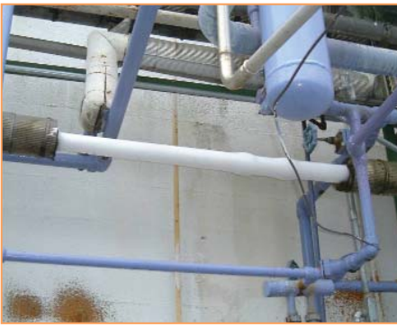
Figure 1: Insulation is missing on this liquid line.
