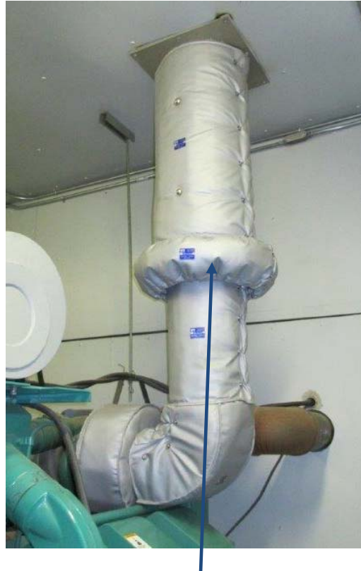
Standard Flange Cover Installed on Engine Exhaust.
